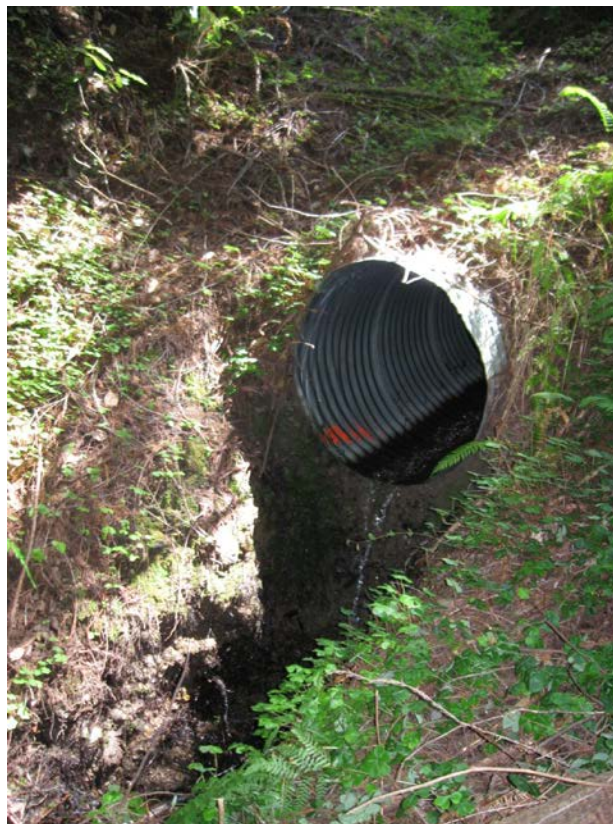
Figure 73. Steel culvert with significant scour at the outlet (shown), as well as diversion potential (not shown) (1-97NTMP-018 MEN).
