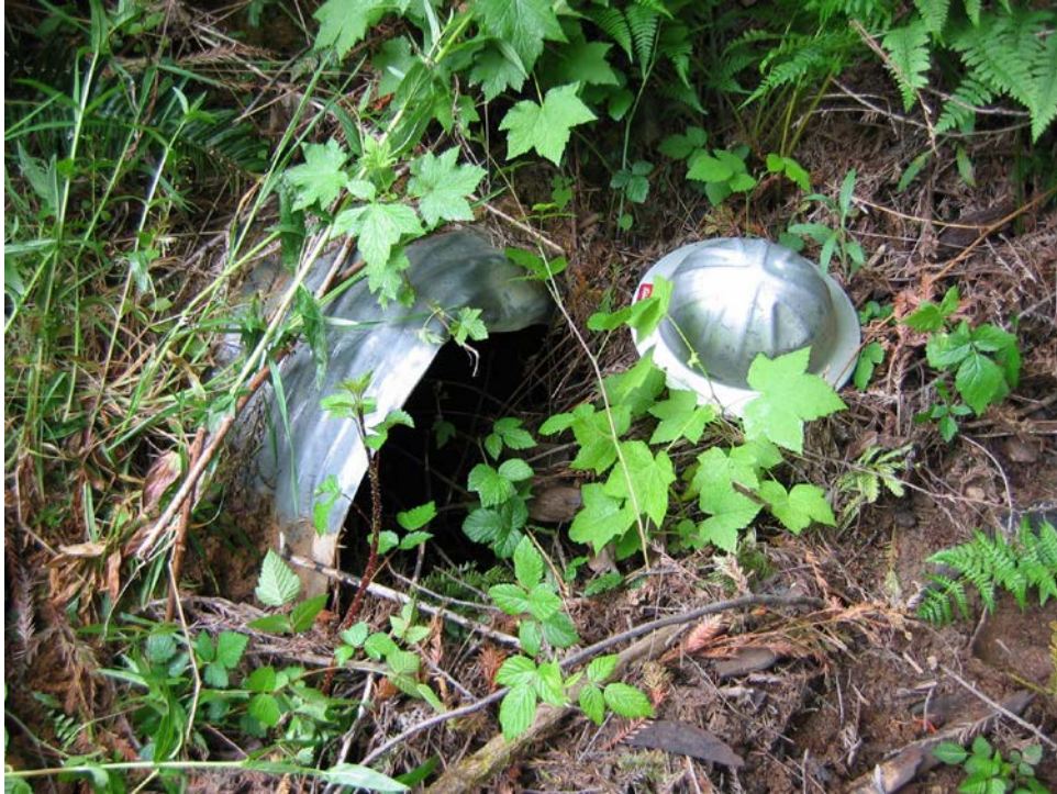
Figure 64. Culvert crossing with sediment and debris blocking more than 30% of the inlet (major problem), THP 1-05-246 HUM, crossing number 1.
