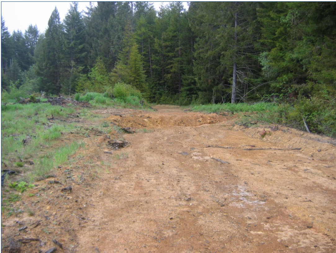
Figure 32. Example of a seasonal road with a properly installed waterbreak (THP in the FORPRIEM sample in Humboldt County).
