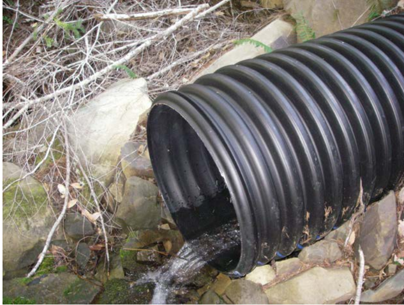
Figure 60. 30-inch corrugated plastic pipe outlet, THP 1-06-107 MEN.
