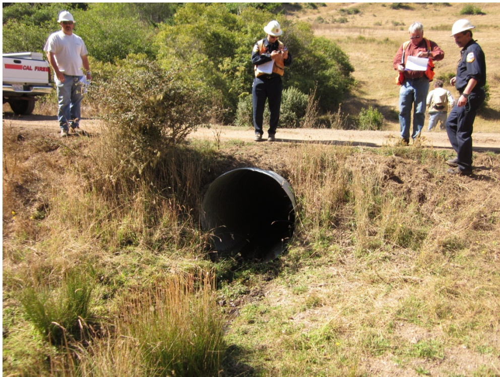
Figure 56. Joint CAL FIRE and NCRWQCB staff inspection of a watercourse crossing evaluated in August 2011 (1-97NTMP-018 MEN; NTO #6).
