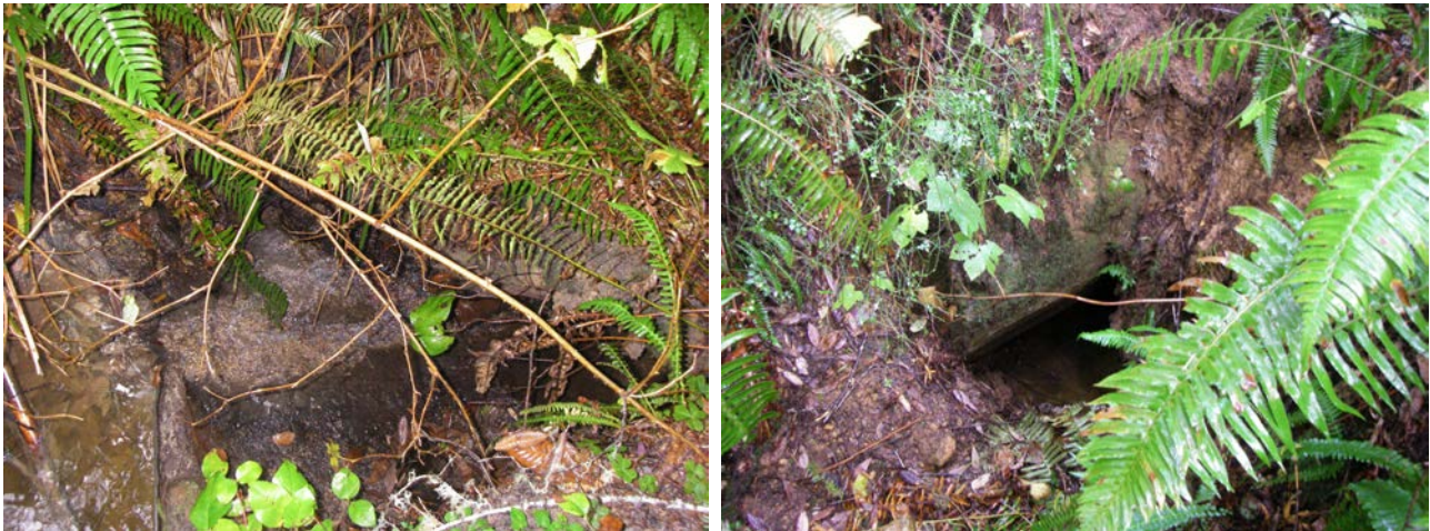
Figure 68. Photos of a Humboldt (log-filled) crossing in the sample from an NTMP-NTO in Mendocino County. The crossing inlet is shown on the left; the outlet is on the right.
