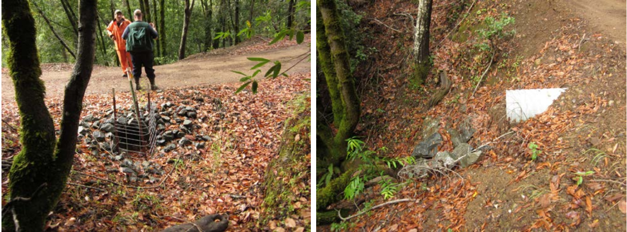
Figure 67. Typical 18 inch culvert (1-97NTMP-038). The crossing inlet is shown on the left; the outlet is on the right.
