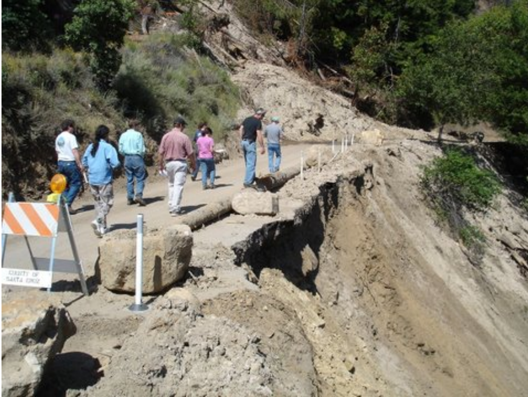
Figure 53. Public roads, such as this road in Santa Cruz County with a major landslide feature, were not included in the FORPRIEM sample.
