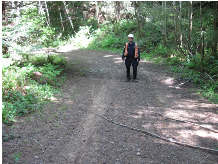
Figure 39. Examples of road segments in the FORPRIEM sample with appropriate road drainage facility spacing and without erosion features.
