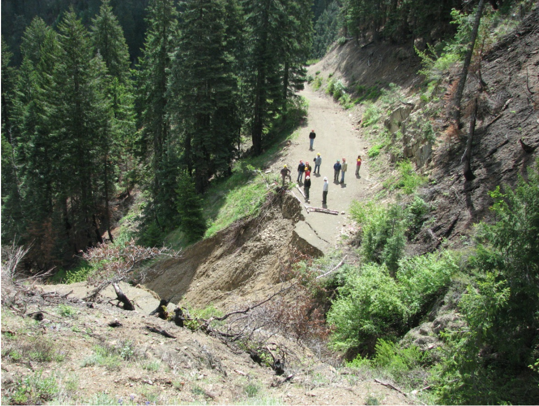
Figure 77. Road fill failure in the Hawkins Creek watershed resulting from the December 2012 storm event (photo from USFS 2013, provided by Juan de la Fuente, Shasta-Trinity National Forest).
