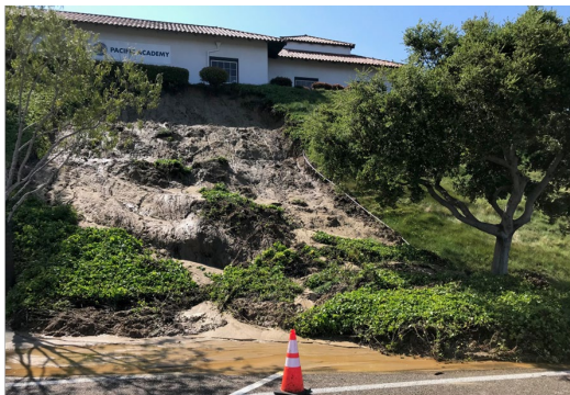
Surficial Slope Failure Caused by Heavy Rain
