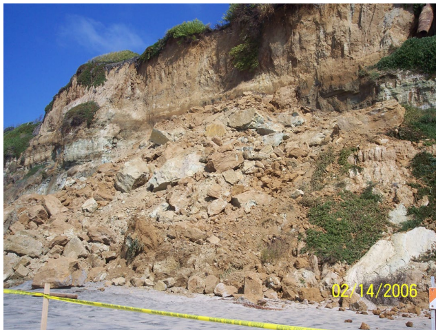
Example of Bluff Failure in Encinitas
