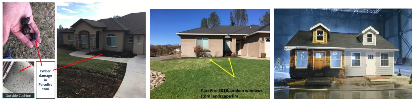
Figure 3. Cracked windows on a newly constructed Paradise home attributed to the use of combustible mulches surrounding the home (left image), cracked windows in Redding attributed to embers igniting combustible mulch and landscape plants (middle image), and new research from IBHS demonstrates the importance of incorporating a noncombustible zone (right image with rock mulch on the right-hand side. See https://disastersafety.org/wildfire/protect-your-home-from-wildfire/ for more details on the research.)
